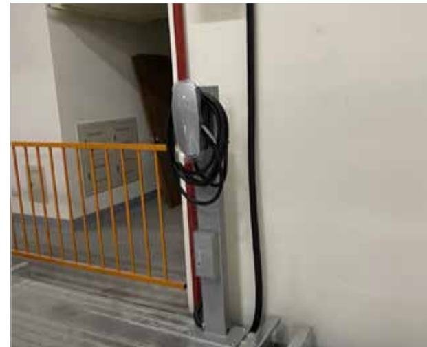
E-Auto-Ladestation E-car charging station
