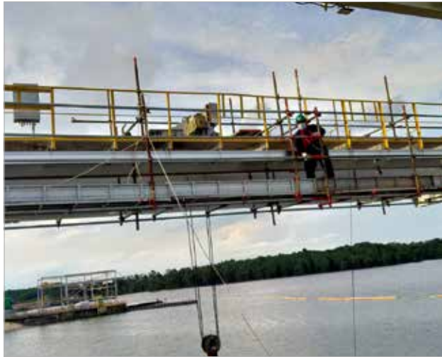
Brückenkran Bridge crane
