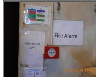
Photo of fire safety equipment DSCN4195.jpg
