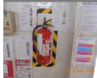
Photo of fire safety equipment DSCN4167.jpg
