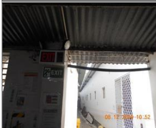
Photo of fire safety equipment DSCN4168.jpg
