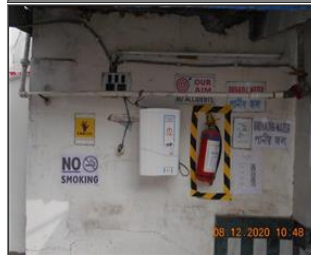
Photo of fire safety equipment DSCN4154.jpg
