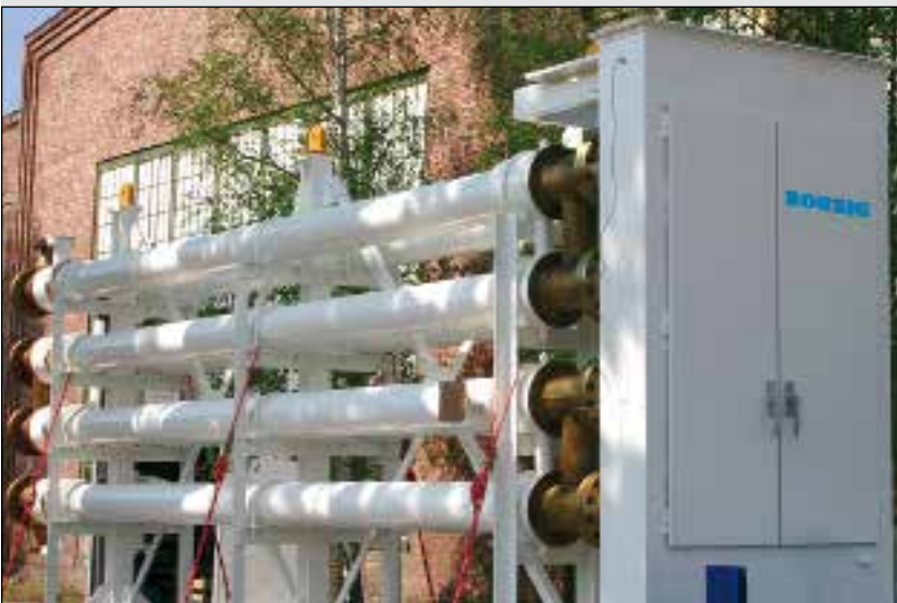
Scraped surface exchanger for fatty acid service
