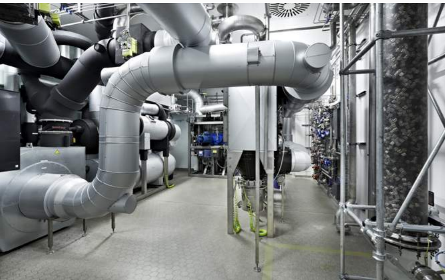
Technical area of a Coating unit with nitrogen circuit and solvent condensation
