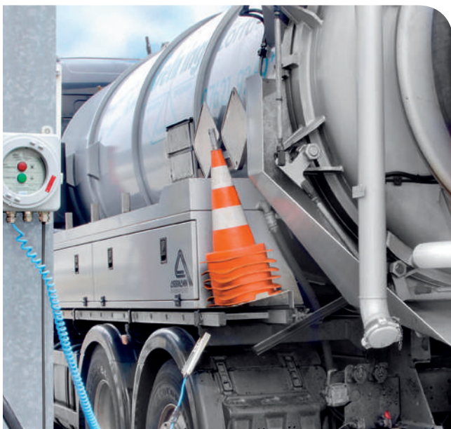
Active grounding for tanker trucks
