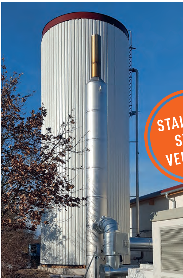
LIPP Thermal Storage Tank, 300 m 3 volume
