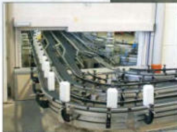
Integration of a fire protection terminal
