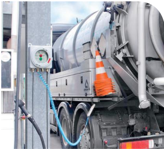
Active grounding for tanker trucks
