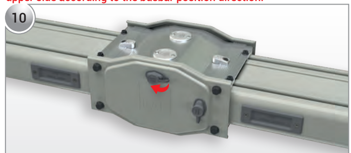
Once the injection is done, plastic lid is placed and installation is completed.
