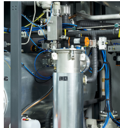
Filter monitoring and drying
